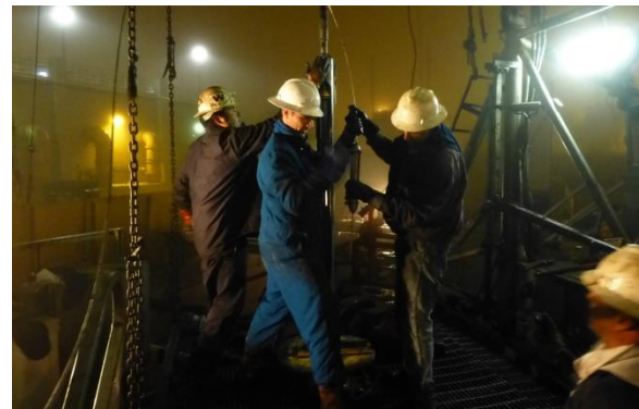
Figure 13. Showing the Fiber Optic Seismic Sensor array during deployment.
